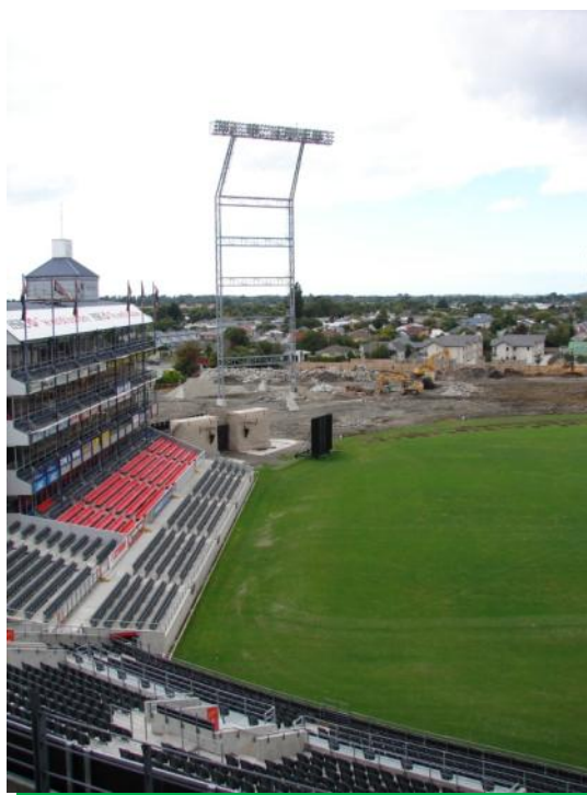
Above: Demolition of the Number 1, 2 and 3 Stands signaled the start of redevelopment works at AMI Stadium
