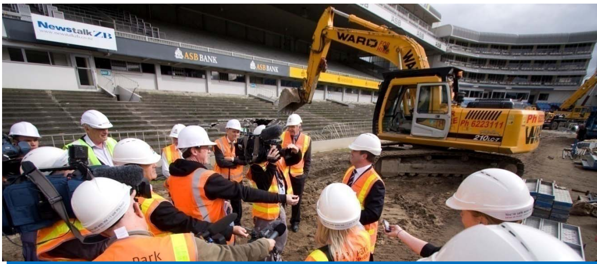
Rugby World Cup Minister Clayton Cosgrove briefs media on the demolition progress at Eden Park as the machinery moves in.
